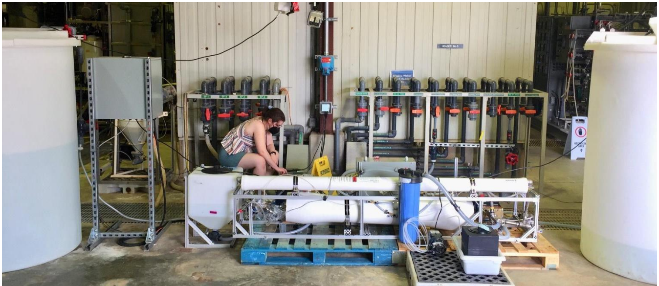
Figure 4: Photograph of the batch RO pilot built at Olin College (Needham, MA) while in operation at the Yuma Desalting Plant in Yuma, AZ. It is pictured separating the plant's brine stream into permeate (left tank) and a more concentrated brine (right tank). The pilot has a permeate production capacity of 5 m 3 /day (0.9 GPM) and maximum operating pressure of 34 bar (500 psi).
